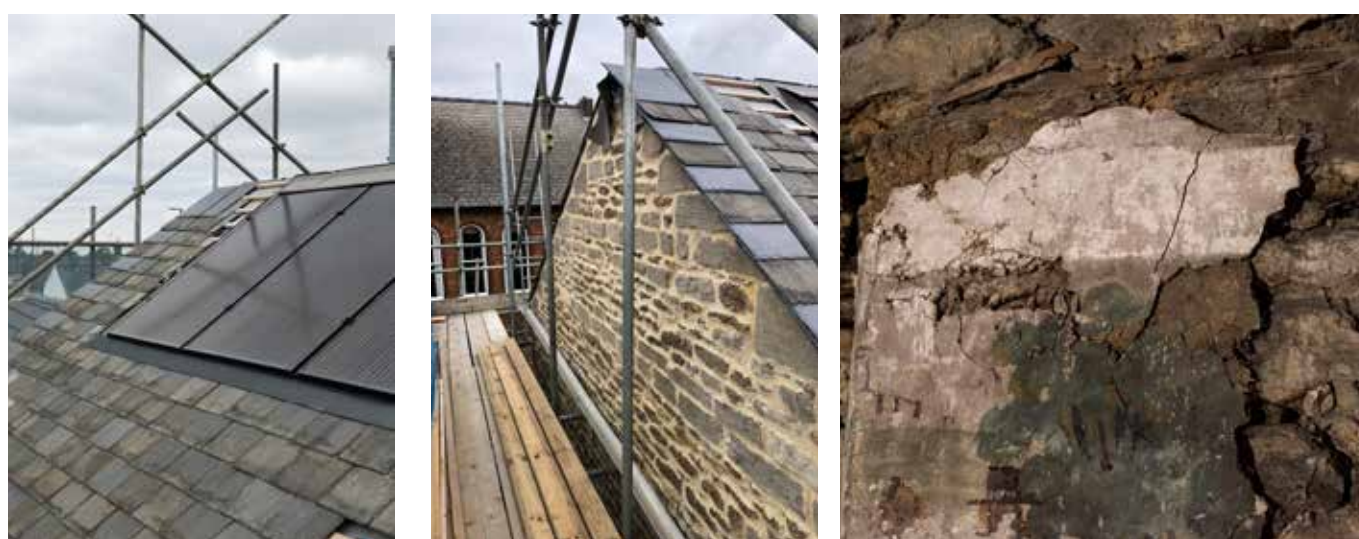
Figs. 47-49. Left, the roof is partially open, the paintings are directly below the opening, a serious cause for concern due to water infiltration. Middle, Guttering also runs along the west wall directly above the painting. Failures to the guttering may cause serious damage to the painting is unmaintained. Right, the rotten lintel behind the painting on the north wall, plans to remove and replace the lintel threaten the survival of the painting.
