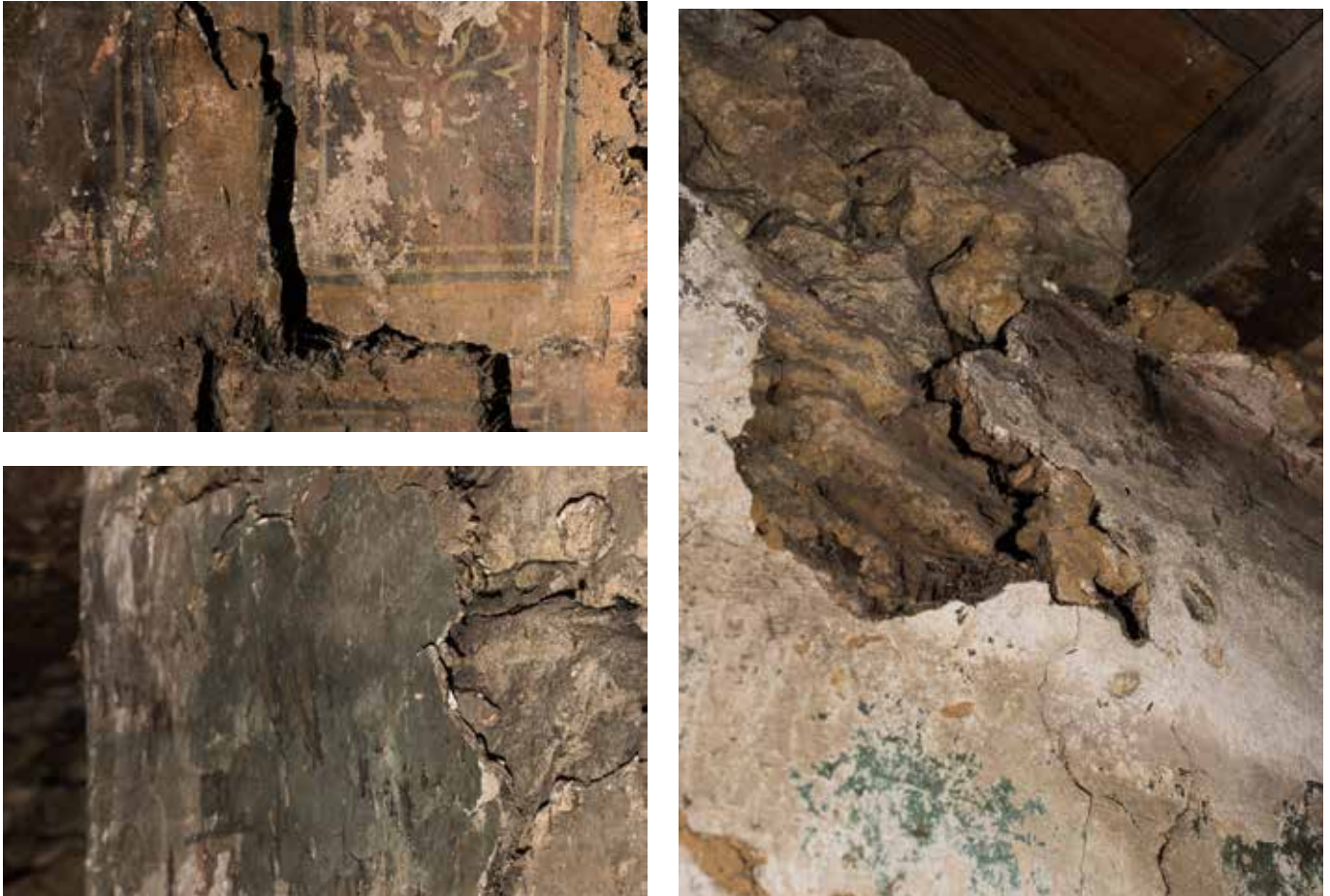
Figs. 35-37. Examples of where de-lamination is occurring. The plaster has separated from the layer beneath leaving a void beneath.
