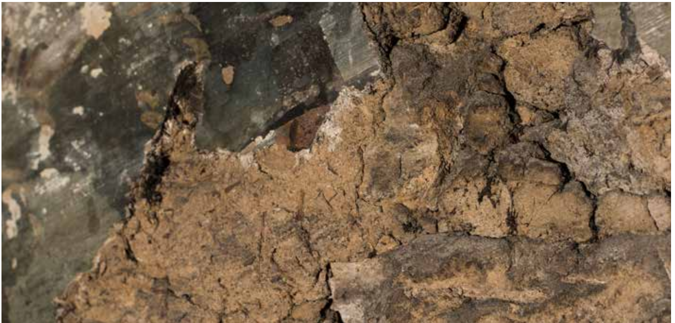
Fig. 24. Left, view showing the rubblestone wall construction onto which, the painted plaster is applied. Upper right, Detail view of the stone support showing through a loss in the painted plaster. Lower right, remains of a wattle and daub ceiling remain at the top of the wall, interestingly this goes behind the painting suggesting it is earlier than the painting itself.
