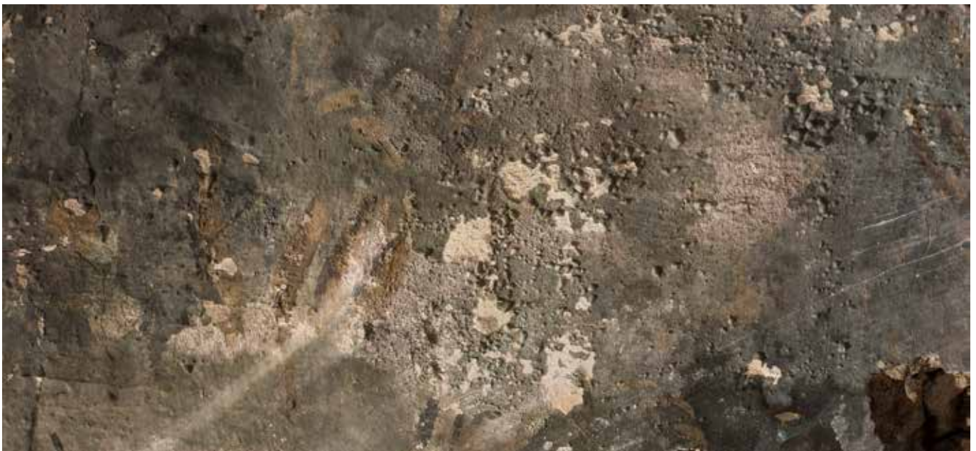
Figs. 41-42. The paint layer appears to have blistered in localised areas. This may be a result of moisture ingress.
