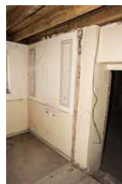
Fig. 51. The room to the south of the paintings. This space will be a kitchen and bathroom. A potential source of liquid and water vapour that could potentially impact the paintings.
