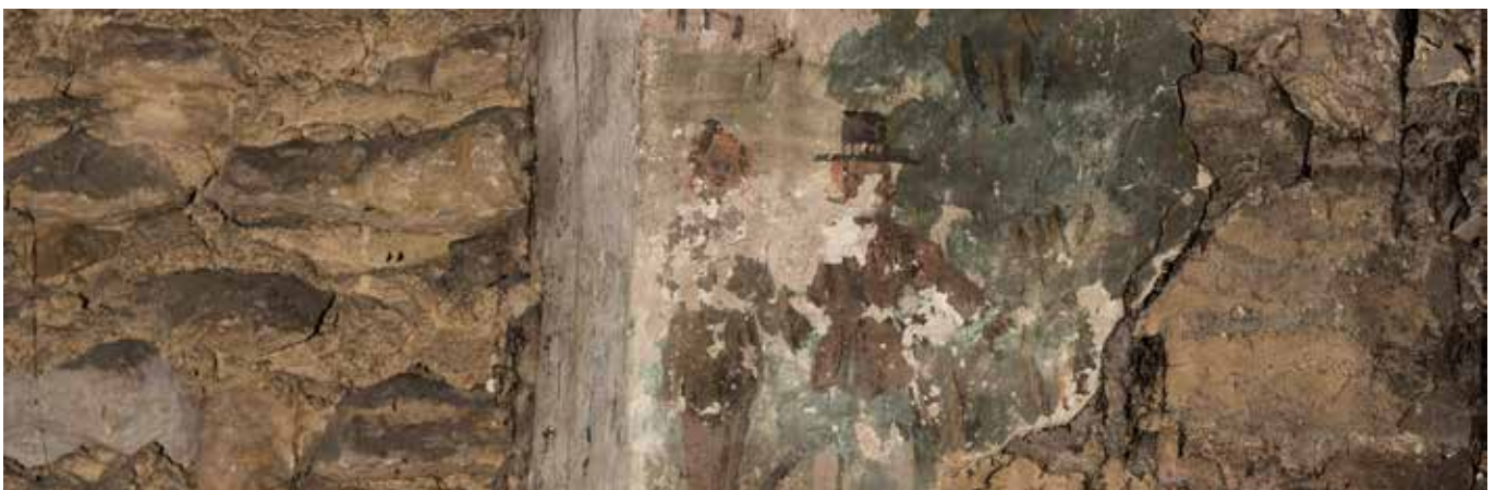
Fig. 38. Extensive plaster loss has occurred leaving only fragmentary remains of the painting on the north wall.
