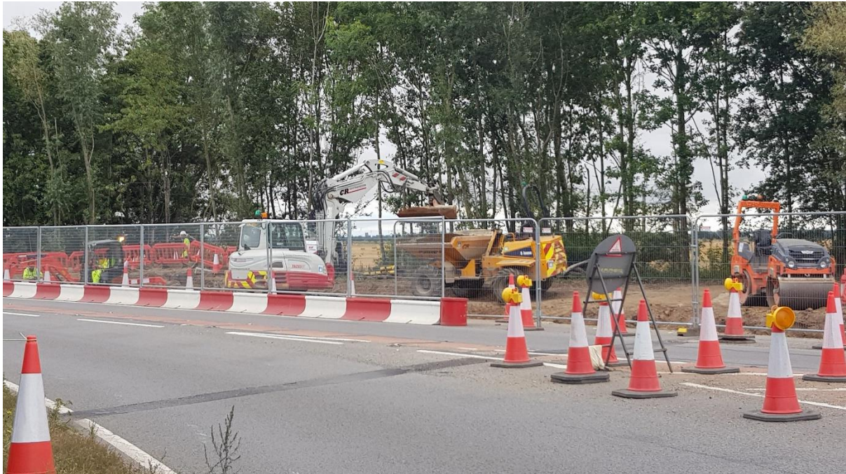
Caption: work taking place to upgrade the Guyhirn junction of the A47
