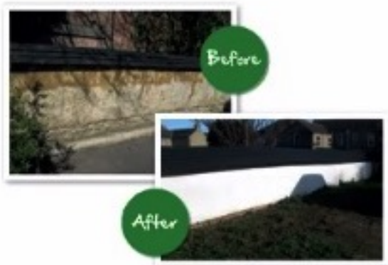
The mud wall at the Black Bull Public House on Market Street before and after it was restored in 2017.
